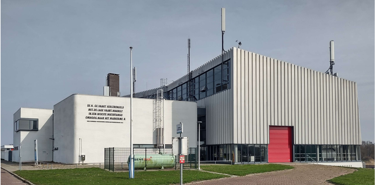
The largest pumping station in Europe
